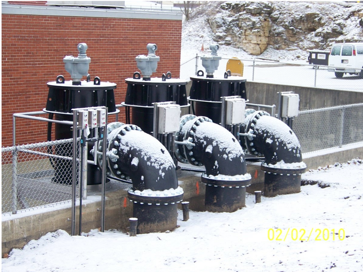
Emergency Effluent Pump Station
